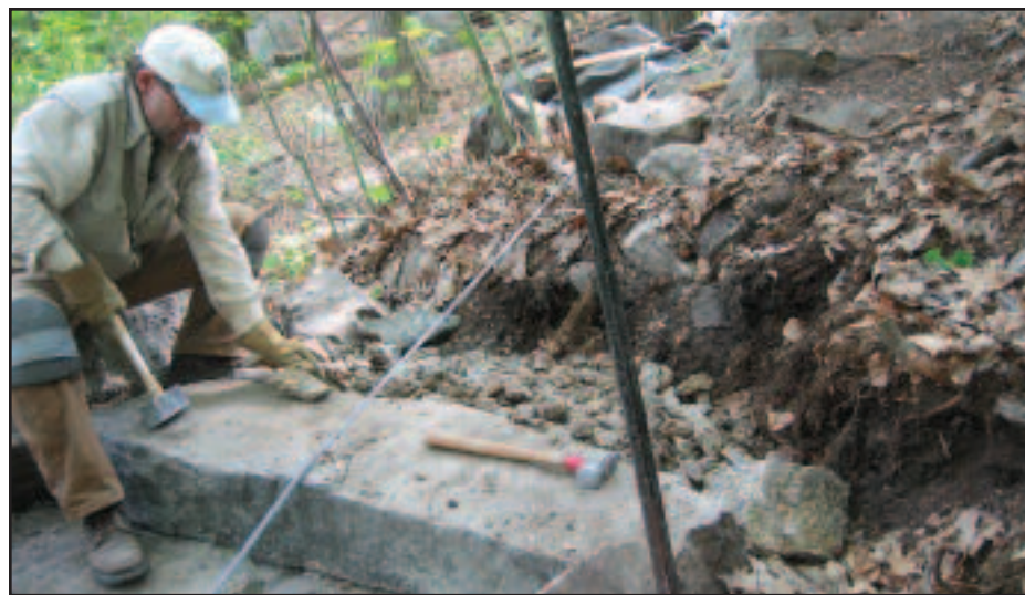
Learn how to install stone steps; just one of many trainings offered by Trail U.
