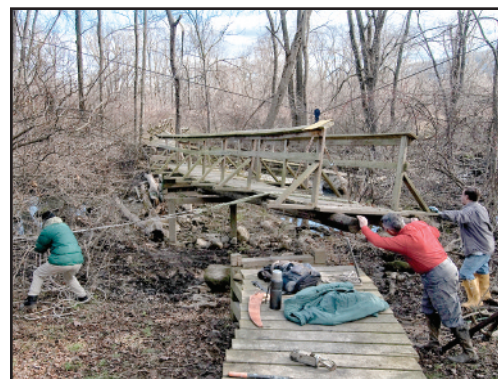
New Jersey Region: A bridge is replaced on the Appalachian Trail along the Pochuck Canal.
